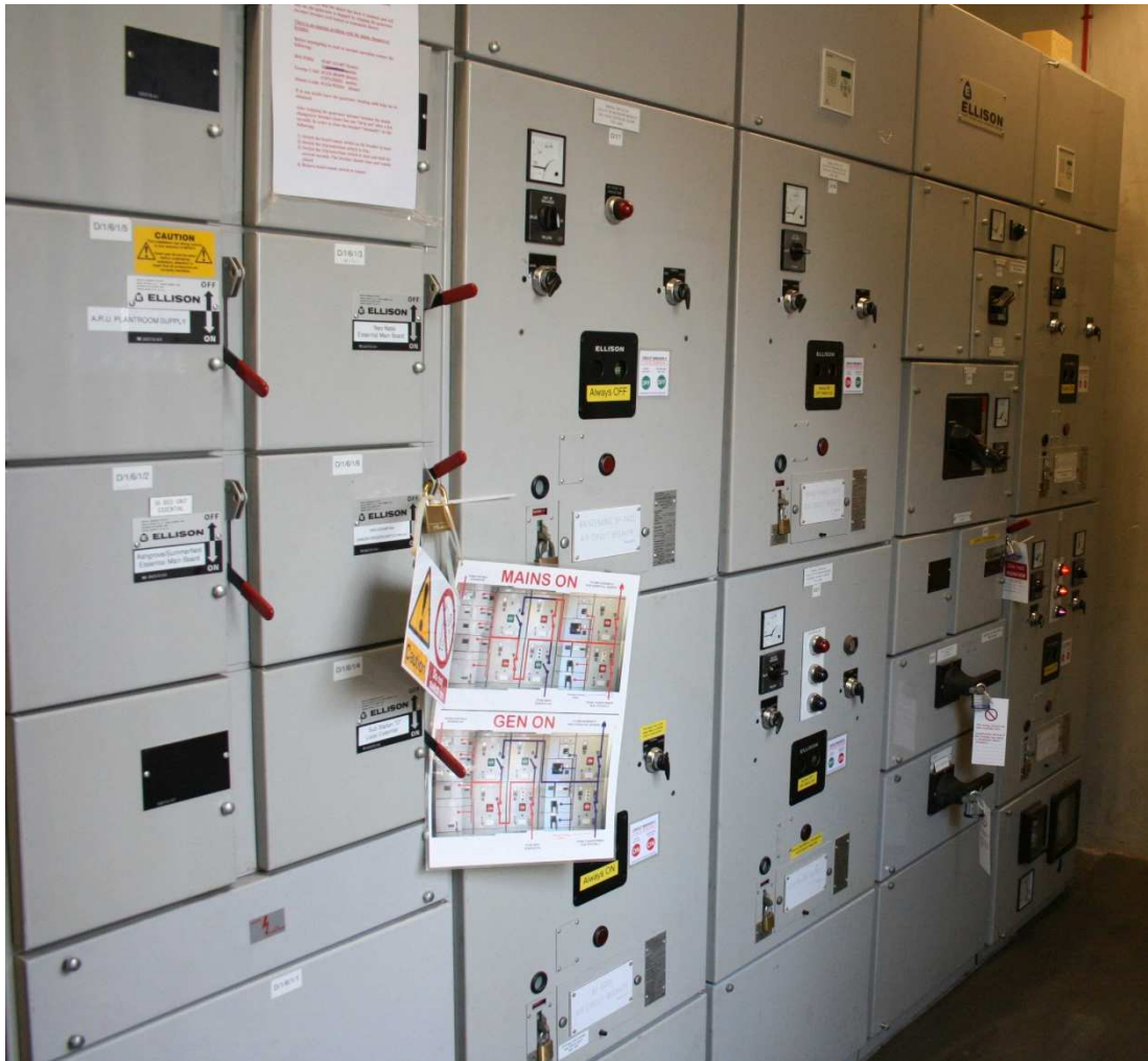
Main switchboard at Aberdeen Hospital requiring ACB retrofits.....
