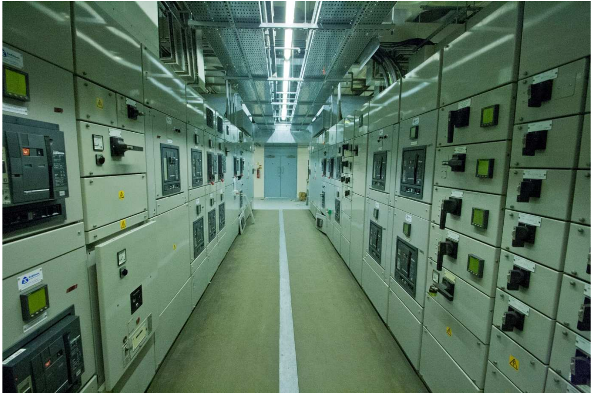
This photograph shows 21 of 43 ACB retrofits completed at a UK data center. In this case Schneider ACBs were utilized.
